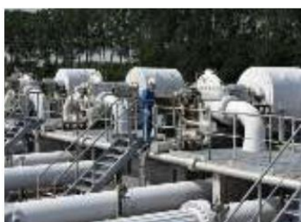
Power Pump Station
